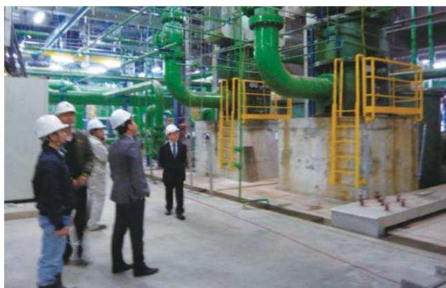
At the Vung Ang Power Plant Division
