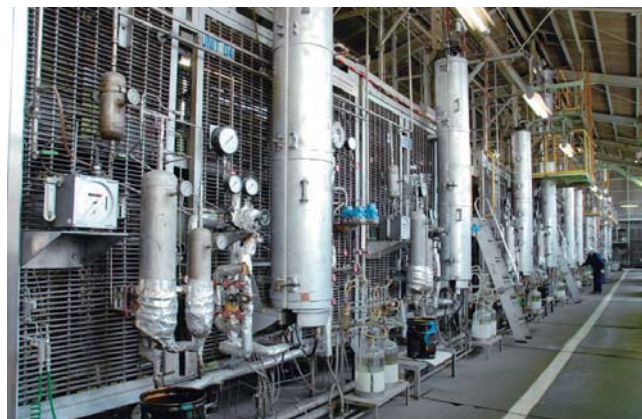
Hydrotreatment pilot plant at JGC Catalysts and Chemicals Ltd.
