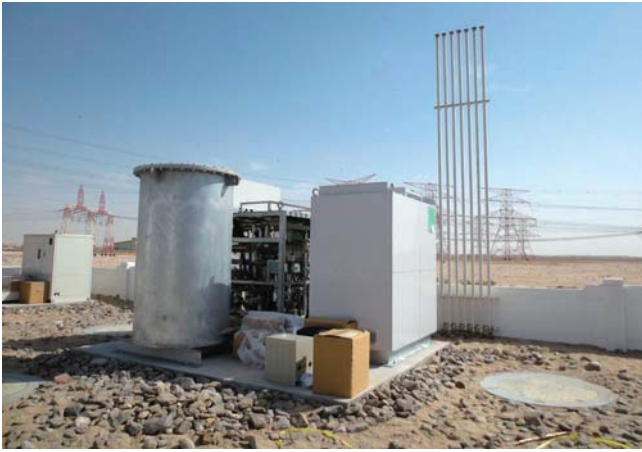
The VRU that was transferred to SS949 (photo provided by JX Nippon Oil & Energy Corporation)
