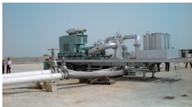
Circulation pump (the pump is mobile)
