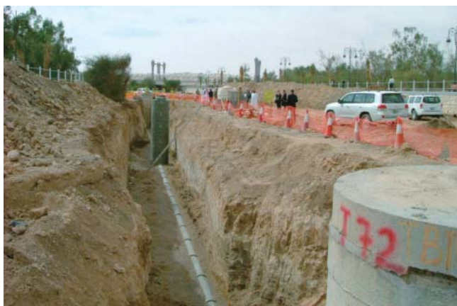
Site of sewage pipe installation work in Al Ain (pipes and manholes before being buried)
