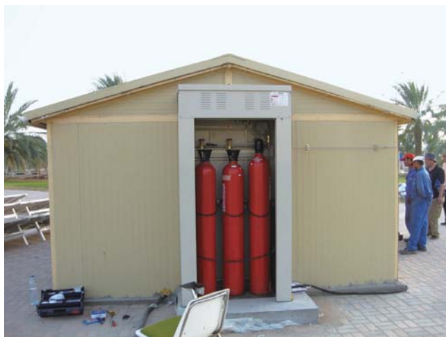
Hydrogen cylinder room
