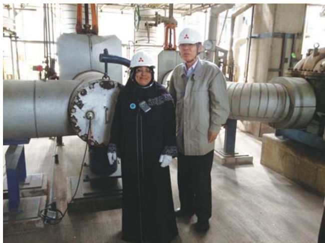
Site tour of the installation of the electrochemical noise device in Japan
