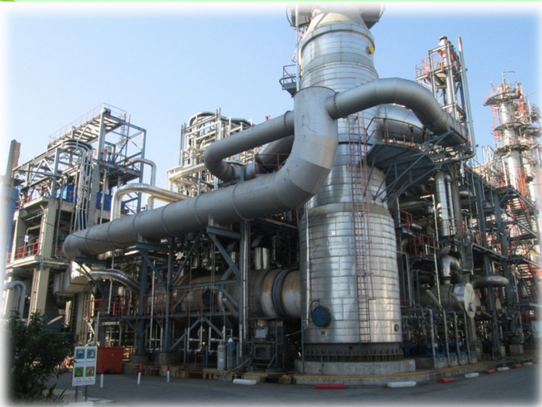
Sulfur Recovery Unit
