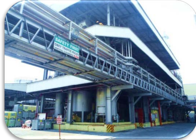
90ML Chemrez Technologies, Inc. Biodiesel Plant Bagumbayan, Quezon City
