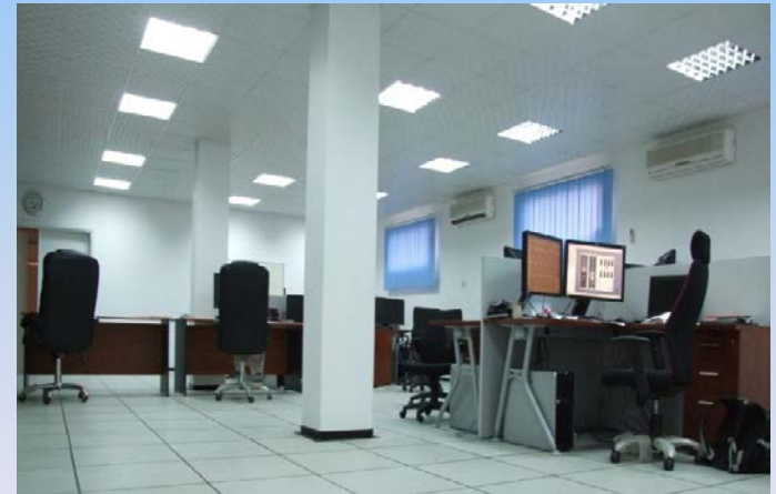
DATA PROCESSING CENTRE
